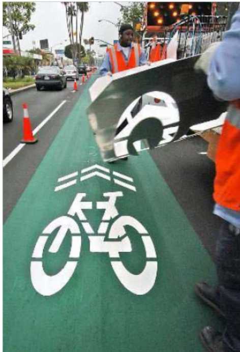
The City of Long Beach Traffic Paint crew apply a 5-foot wide green lane for the first "sharrow," or new Shared Lane Marking, an arrow-like design painted on the roadway to mark a bicycling route along 2nd Street in Belmont Shore between Livingston Drive and Bay Shore Avenue on Thursday. (Diandra Jay/Staff Photographer)
